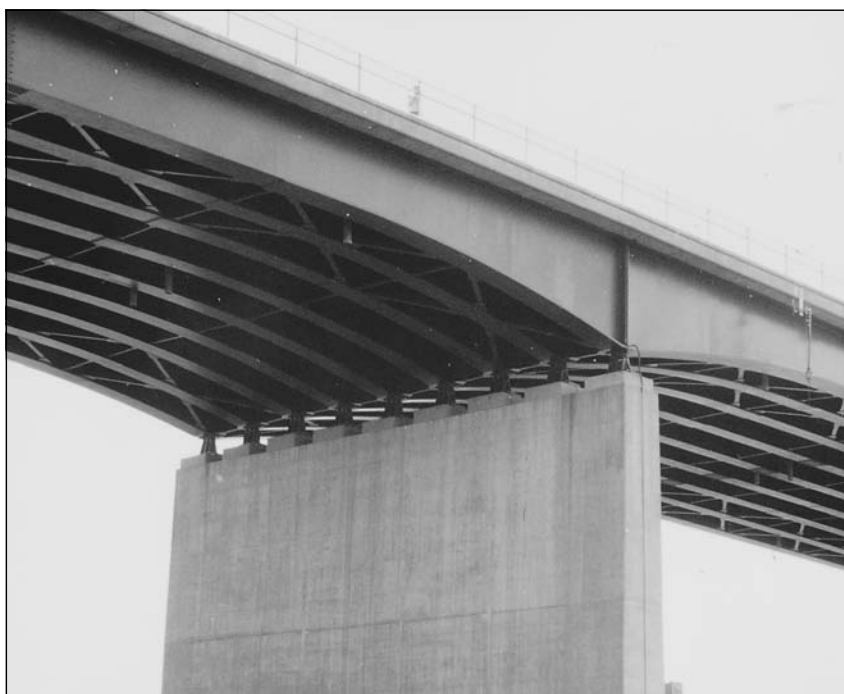
Figure 3.1 A haunched plate girder economizes the amount of steel used for long spans.
