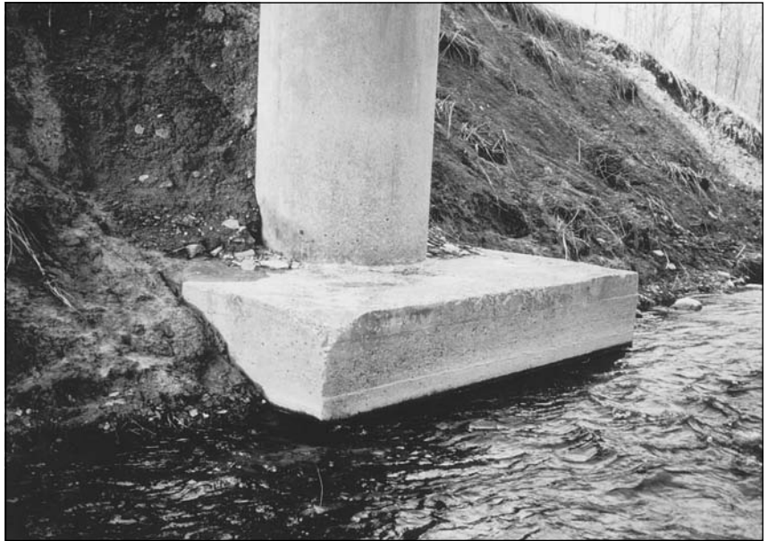
Figure 4.16 An exposed pier footing shows evidence of undermining.
