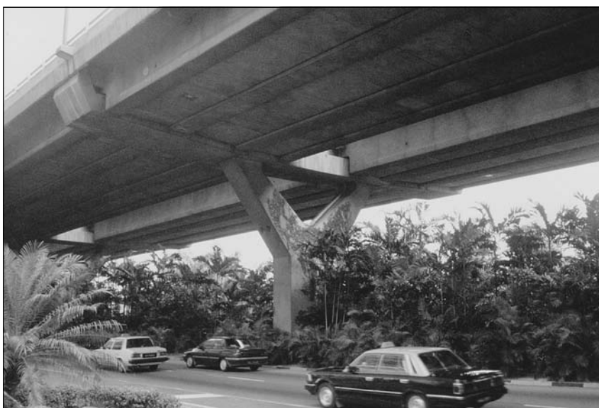
Figure 3.50 A prestressed concrete bridge carries dual roadways over a busy underpass in Singapore.
