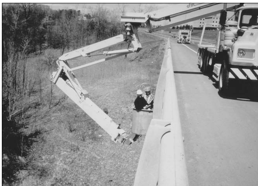
Figure 3.57 A bucket snooper is used to inspect the underside of bridge over water.
