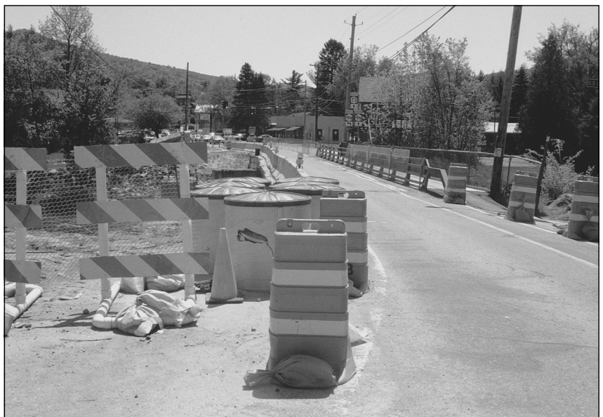
Figure 5.6 Maintenance of traffic devices include drums and break-away barricades.
