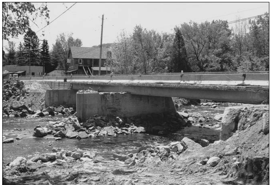
Figure 4.11 It's time for this solid wall pier, located in a stream crossing, to be replaced.
