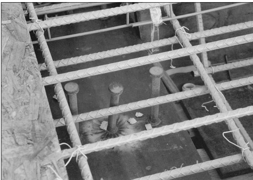
Figure 3.30 A shear stud installed at the top flange of a plate girder. Shear connectors are the key ingredient to preventing slippage and creating composite action.
